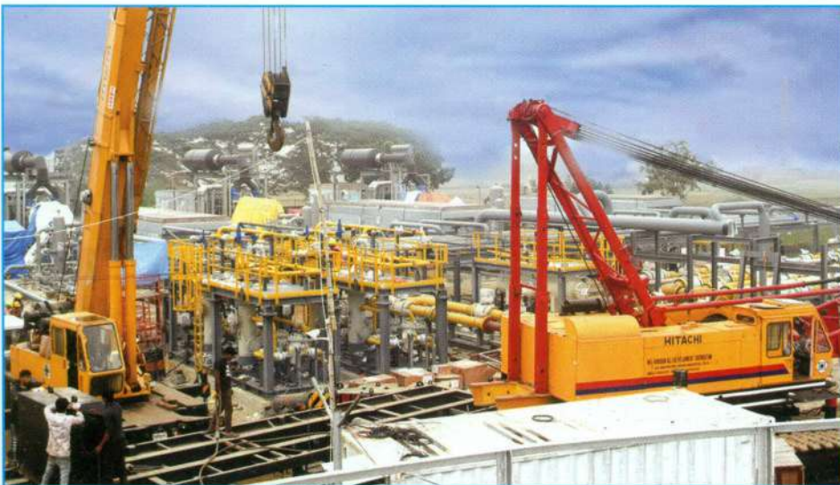
Installation works of Gas Compressor is in progress at Titas Gas Field.
