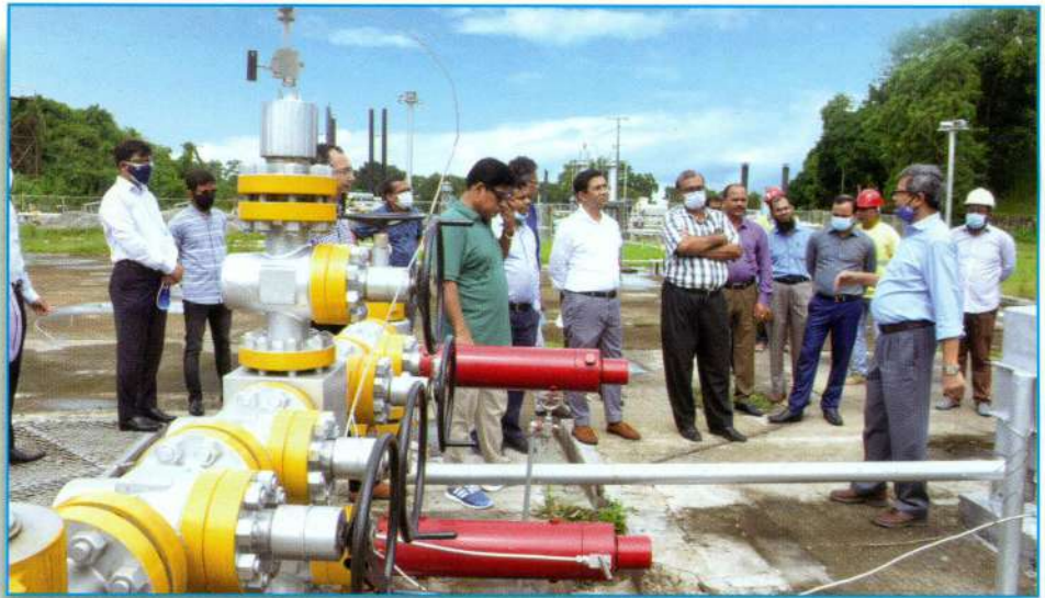
Mr. Abu Hena Md. Rahmatul Muneem, Chairman, NBR & past Chairman, BGFCL board visiting well site & Gas process plant at Habiganj Gas Field.
